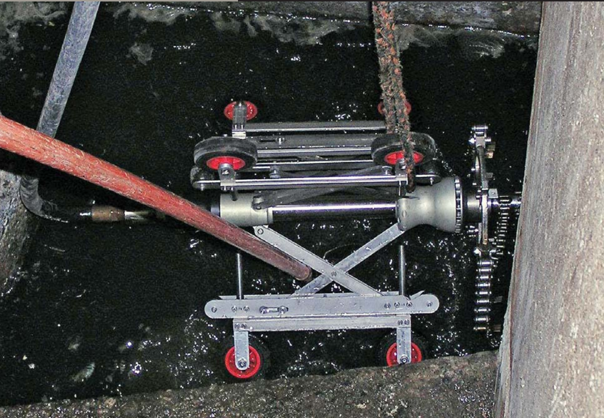
The Turbo III chain cutter helps clear roots from pipes such as this 30-inch sanitary sewer. (Photos courtesy of Ypsilanti Community Utilities Authority)
