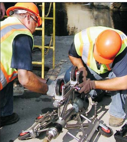
Line service technicians Tom Everard (left) and Ryan Stetler adjust the expandable frame on the cutter.
